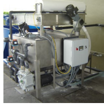
Transit company has long history using CF Systems for oily wash water treatment
